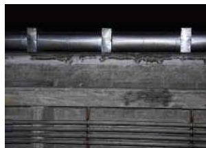
visible imagery *Overhang part of a concrete bridge with multiple main girders
